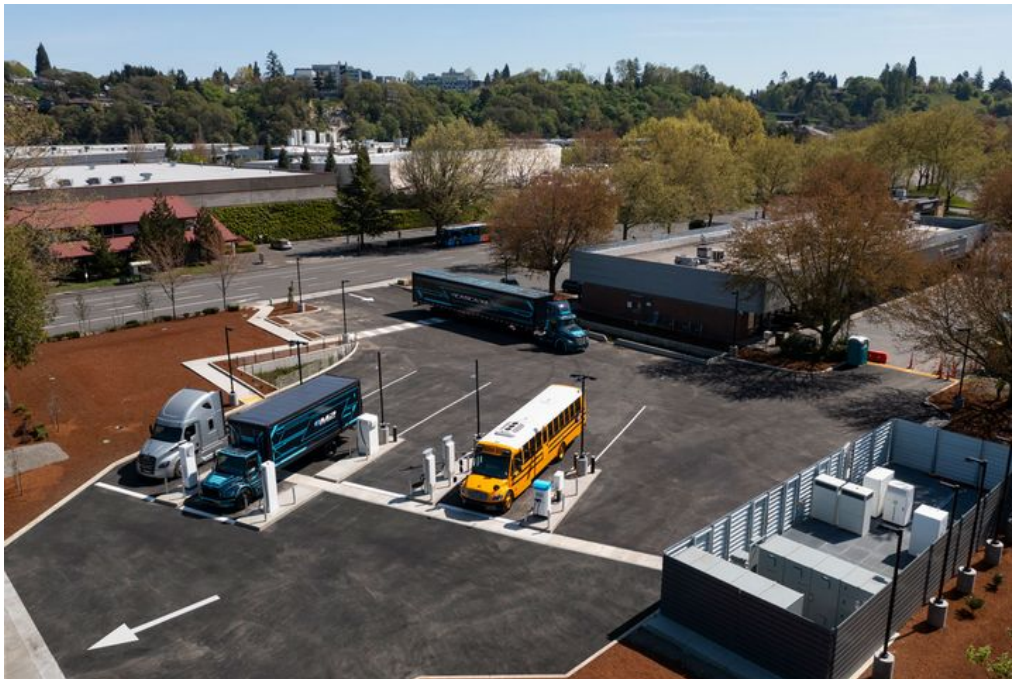
Figure 1. Electric Island Heavy Duty Vehicle Charging Station, Portland, Oregon
