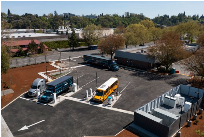
Figure 8-1. Electric Island Heavy Duty Vehicle Charging Station, Portland, Oregon
