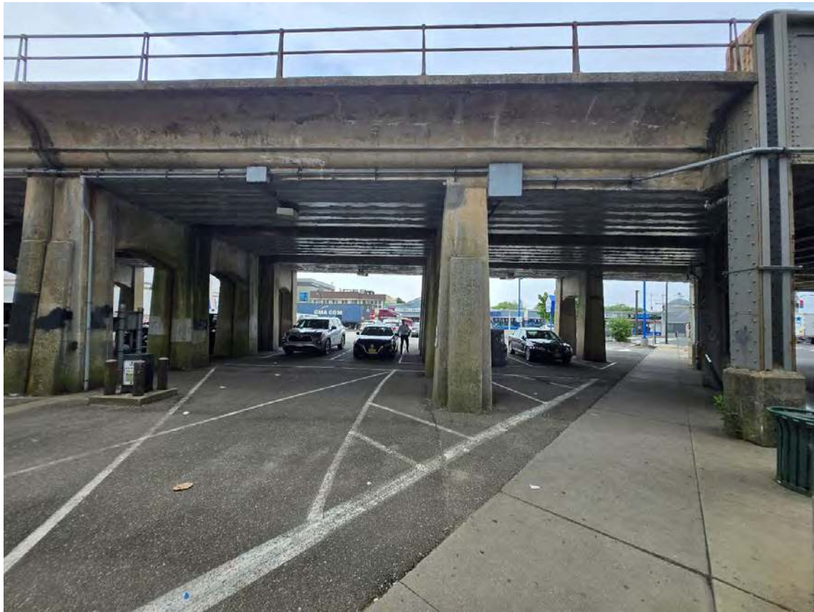
Figure 27: Current conditions of Stanchions at Lynbrook Train Station.
